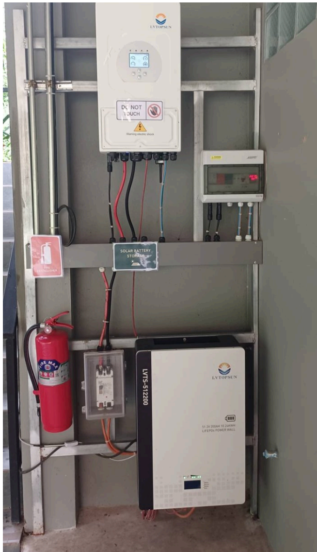
Existing: one battery, fire extinguisher and DC breaker box in the bay
