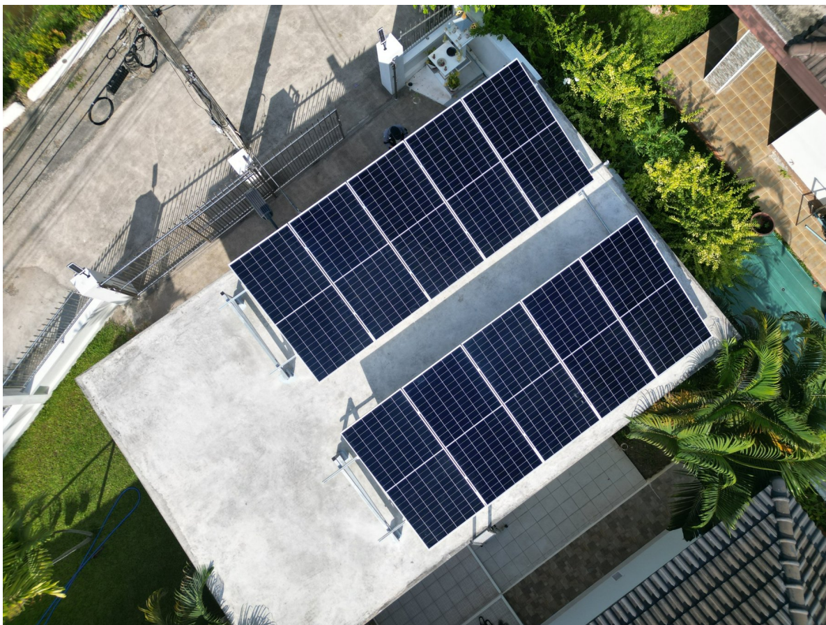
Drone view of the installation: two arrays of five modules each on a flat concrete roof slab.
