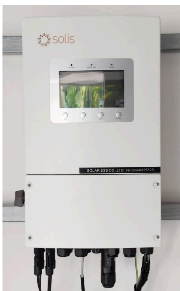
Solis hybrid inverter. The DC switch is the black knob on its left side.
