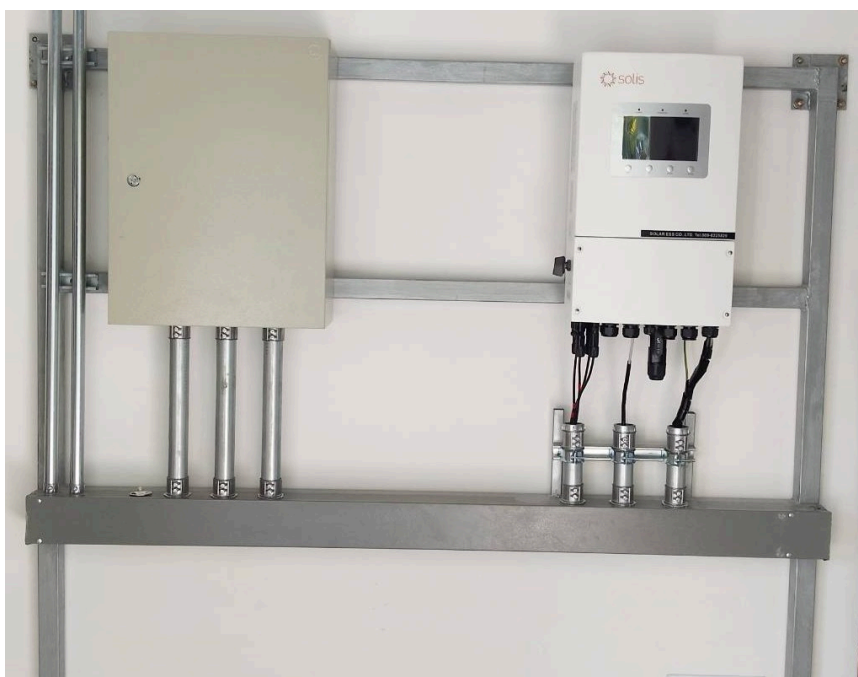
Control cabinet (left) and Solis hybrid inverter (right) on the galvanized steel frame.
