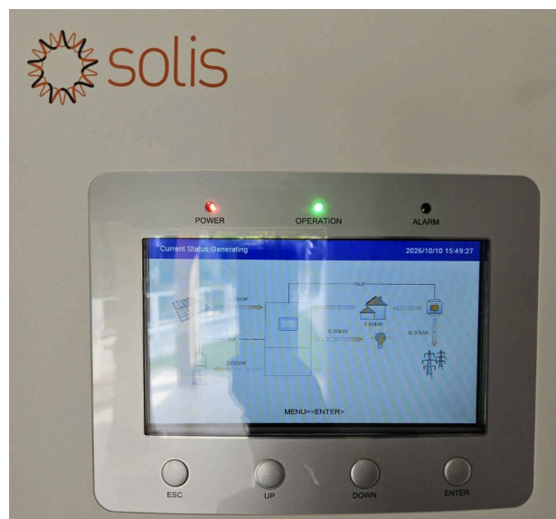
Inverter display and indicator lights during normal operation.
