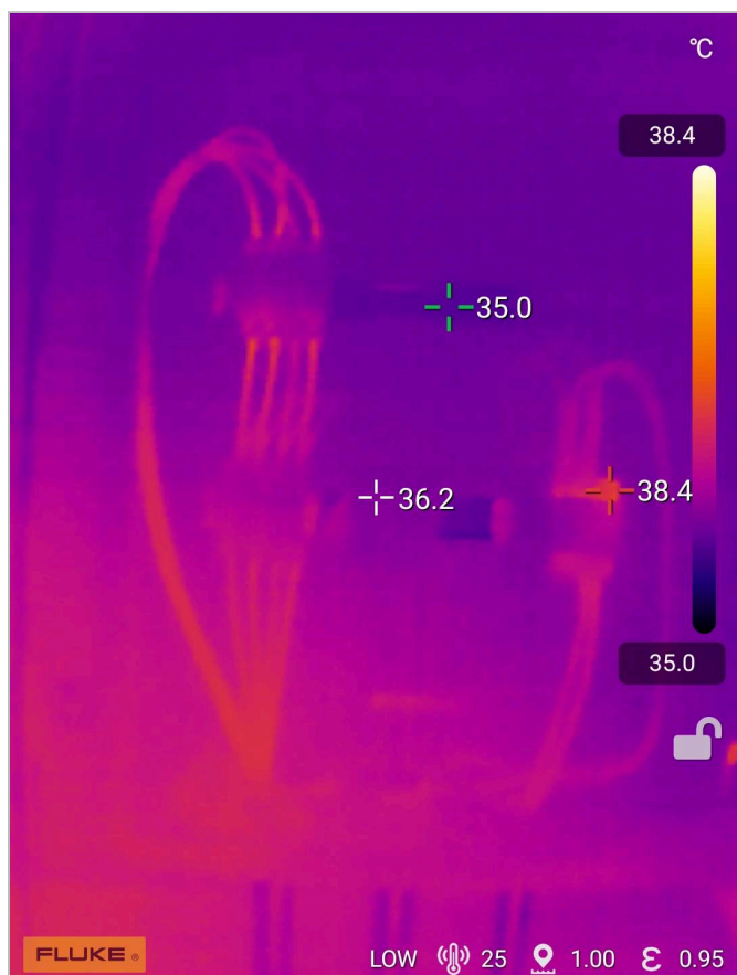
Thermal image of the control cabinet (Fluke, emissivity 0.95).
